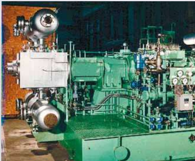
Process gas cooling
