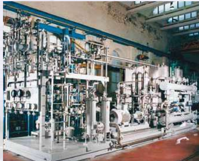
Compressed air cooling
